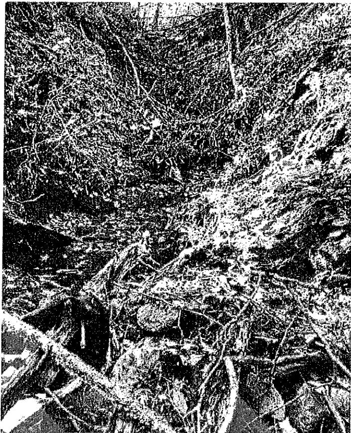
Debris Filled Gully
