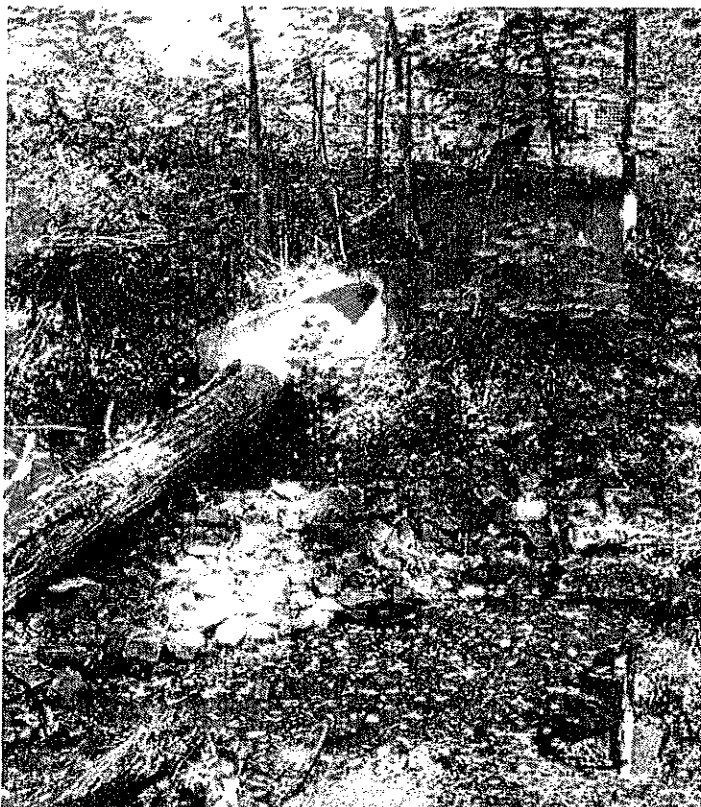
Culvert Behind Squire Hill Pump Station w/ No Rip Rap
