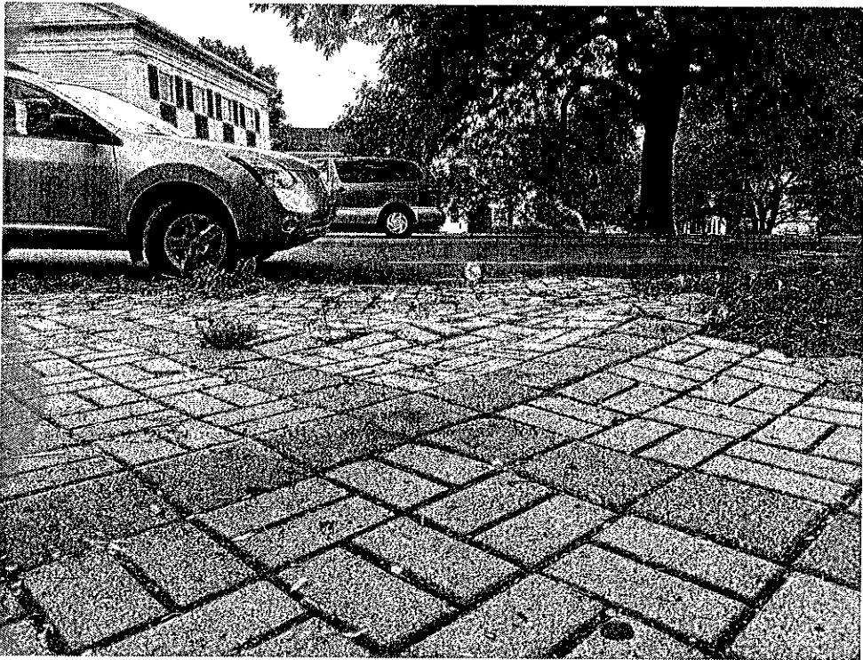
Figure 6. Heaving of pavers causing trip hazards.
