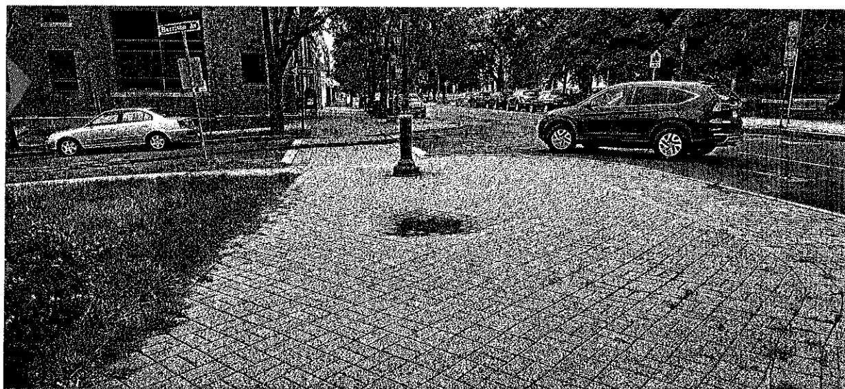
Figure 10. Uneven pavement settlement causing ponding.
