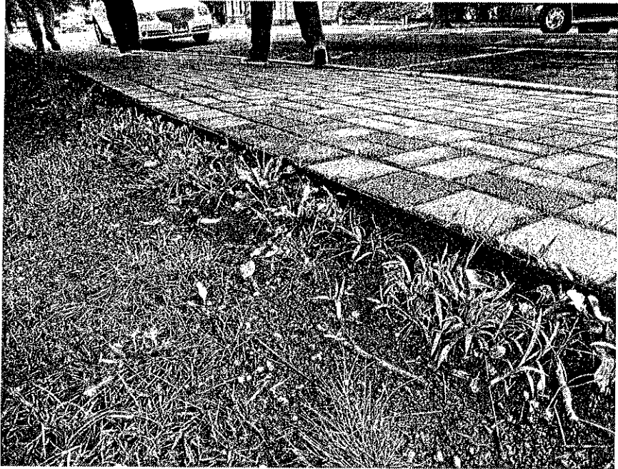
Figure 5. Erosion at back of sidewalk.
