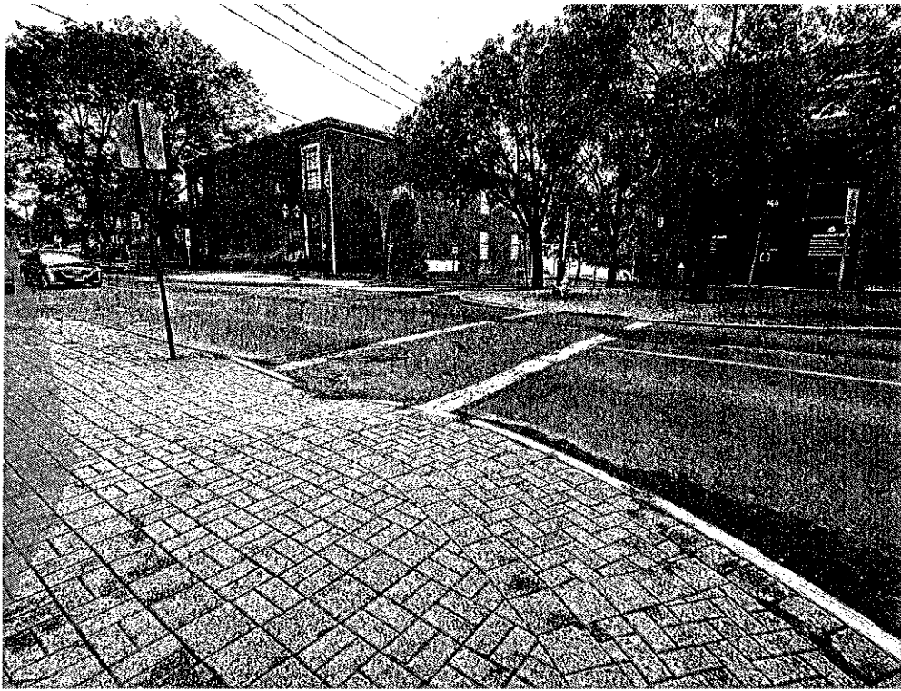
Figure 1. Representative photo of non-ADA compliant sidewalk ramps and crosswalks in poor condition.
