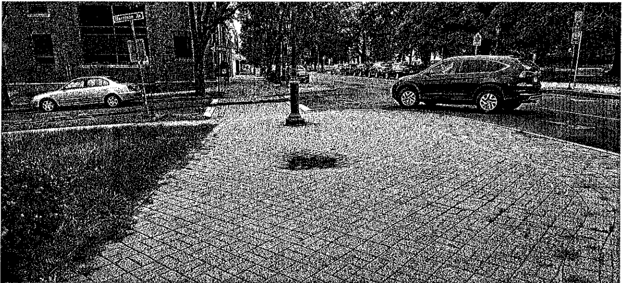
Figure 10. Uneven pavement settlement causing ponding.
