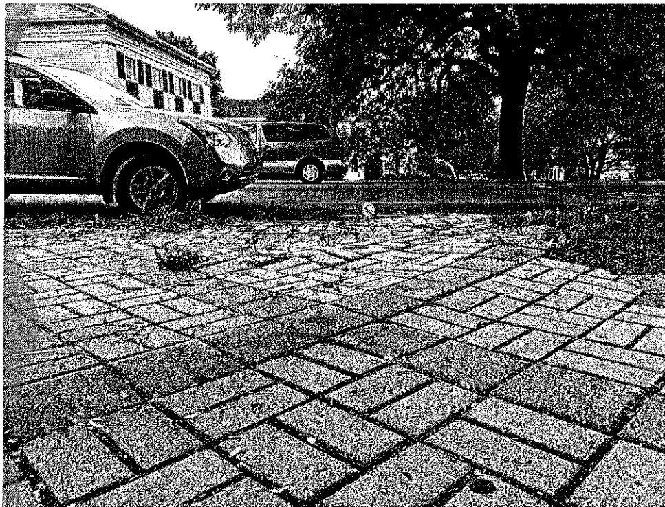
Figure 6. Heaving of pavers causing trip hazards.
