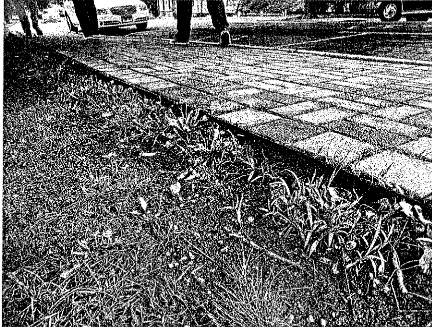
Figure 5. Erosion at back of sidewalk.
