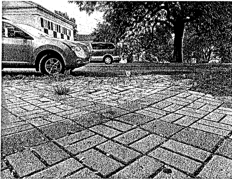
Figure 6. Heaving of pavers causing trip hazards.
