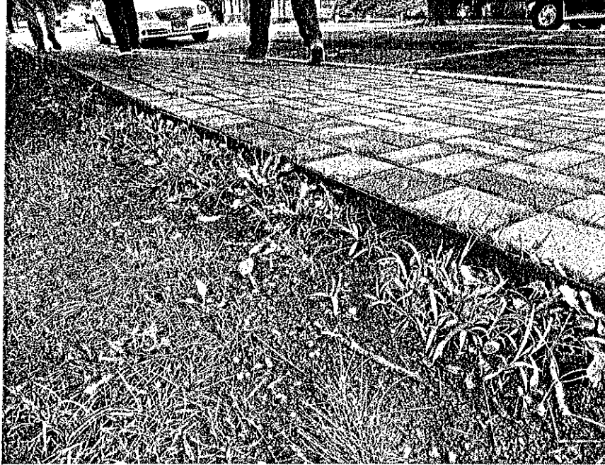
Figure 5. Erosion at back of sidewalk.
