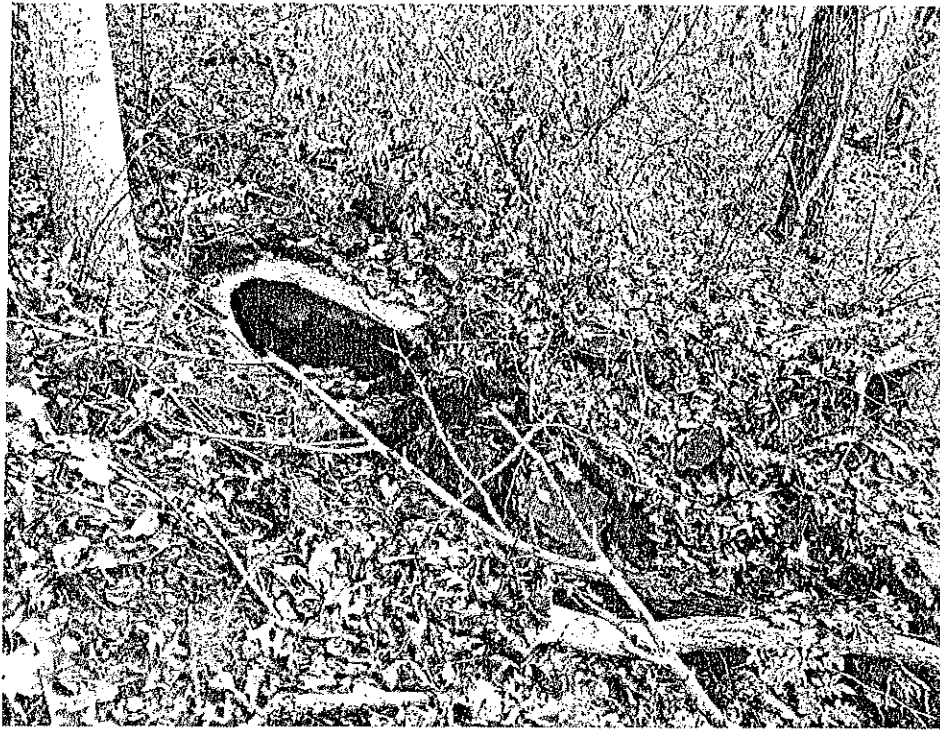
Photo 3: outlet protection (reconfigure with existing rip-rap)
