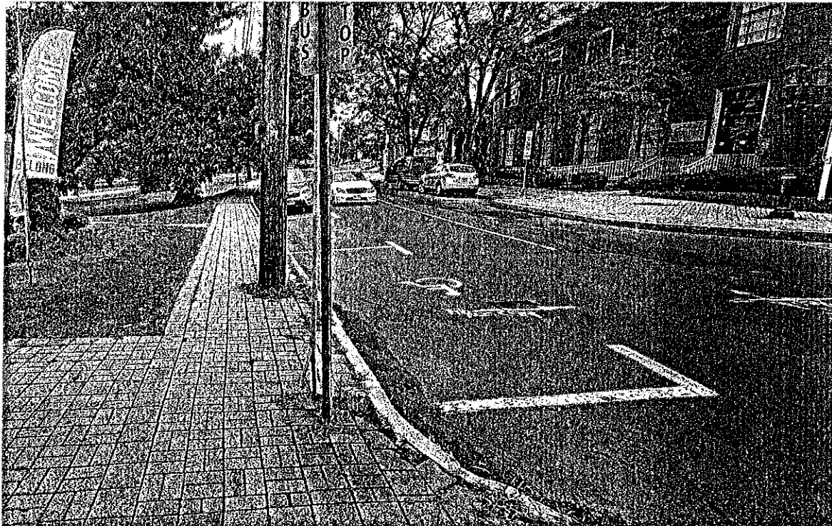
Figure 2. Non-ADA compliant handicap parking spaces.
