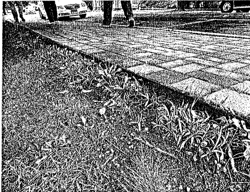
Figure 5. Erosion at back of sidewalk.
