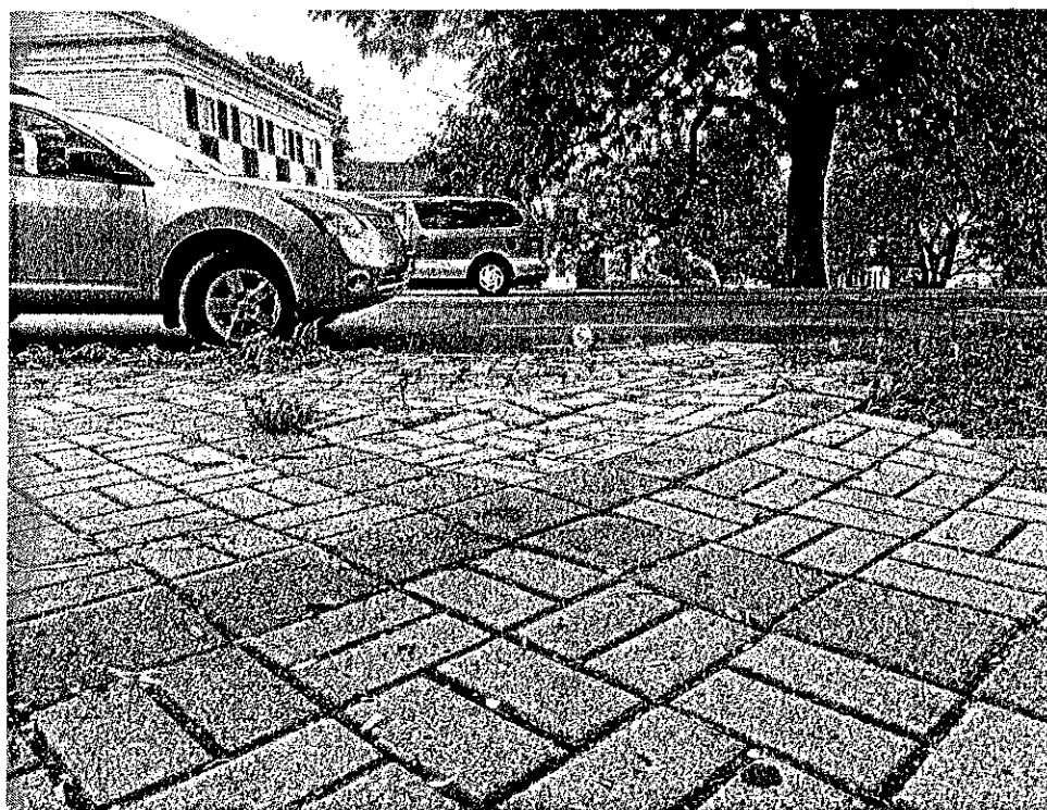
Figure 6. Heaving of pavers causing trip hazards.
