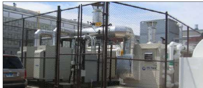
Branford High School – tri-generation unit
