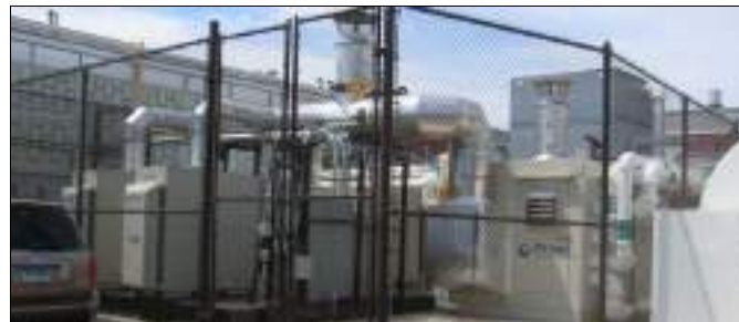
Branford High School – tri-generation unit
