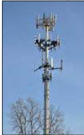
Common Tower With No Camouflage
