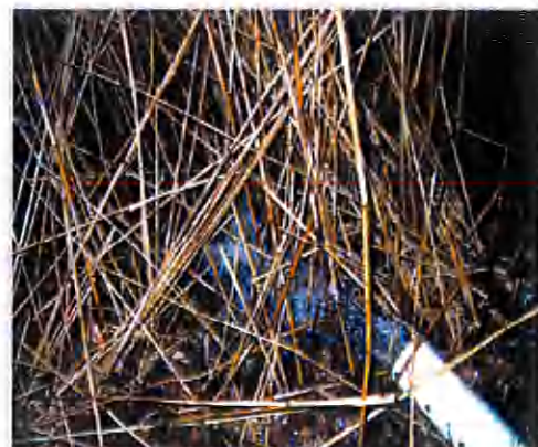
Figure 2-7. PVC pipe draining water from ledge under basement into marsh during a rainstorm (April 2004).
